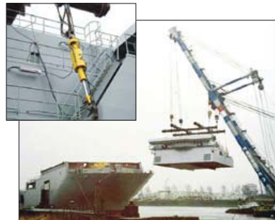
▲ Perfectly synchronised balance: Naval ship superstructure weighing over 600 tons placed on the hull using Enerpac's hydraulic SyncHoist.
