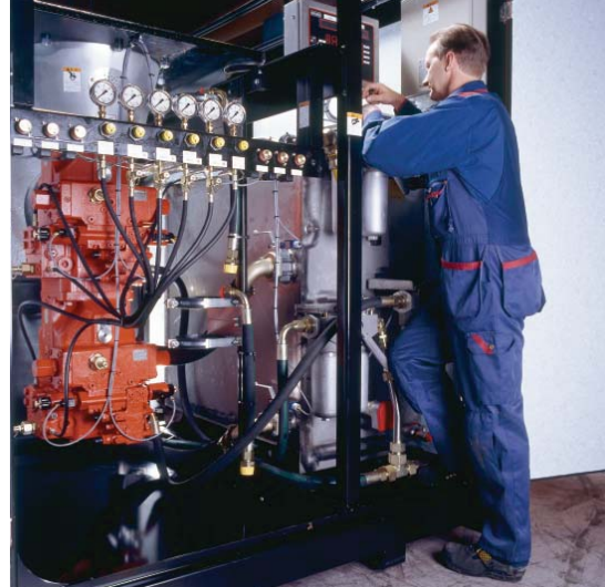
PEC cabinet with tandem mounted pumps
