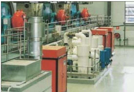
Pulp & Paper. Wash presses, Finland.
